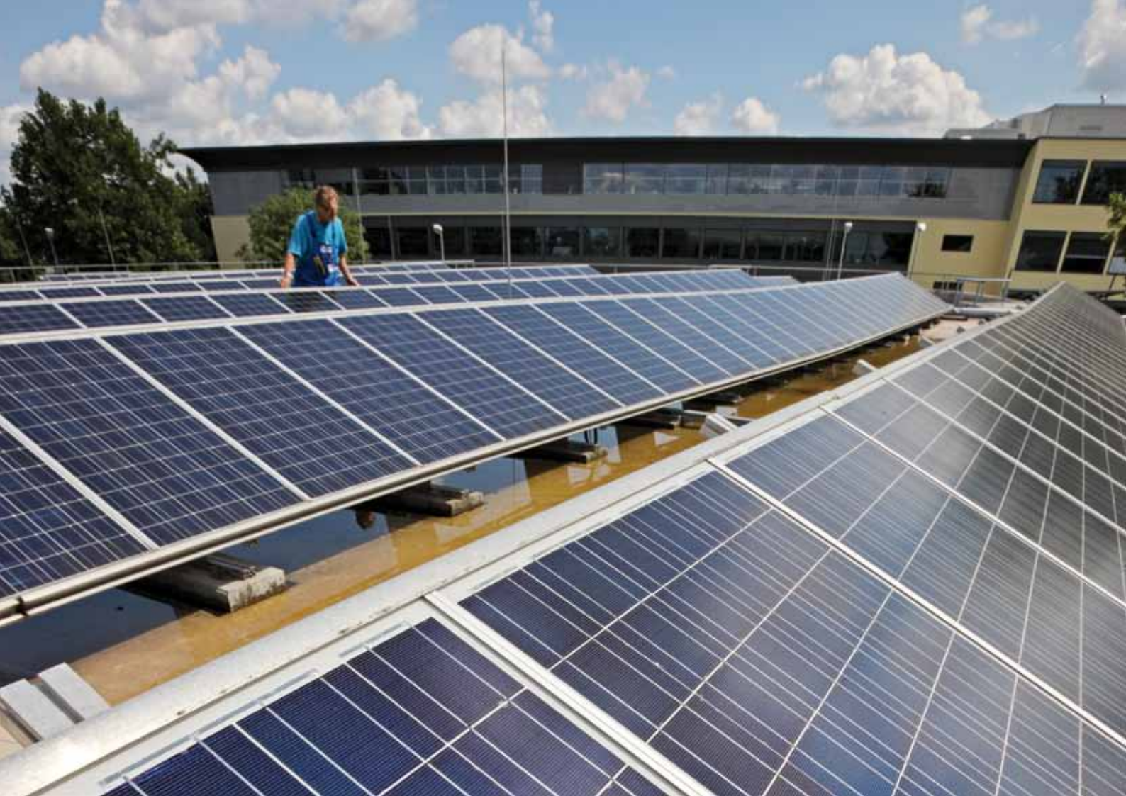
Visual inspection of the solar modules on the roof of Building G.
